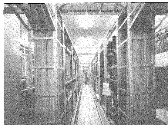
Figure 10—View of 2 of the 21 rows of equipment in the Oslo automatic toll exchange.
