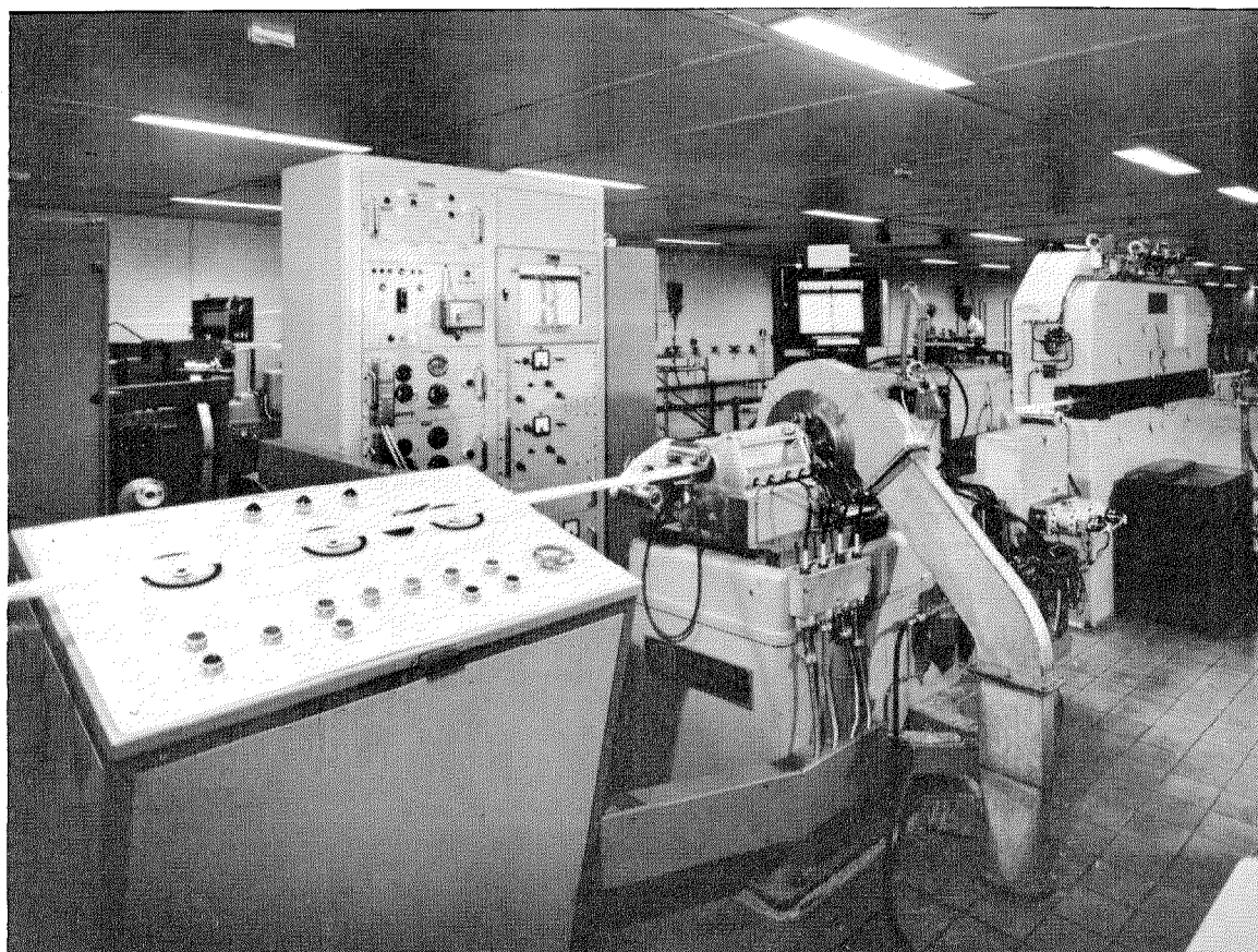
Figure 8—One of the core-shaving machines. At its extreme right is a caterpillar hauler for bringing the core to the shaving head within the circular blower casing where the polythene shavings are exhausted into the ducting going down through the floor. Up against this is the eccentricity head which, with the two racks of equipment behind the line, servo-controls the cutter axis about the conductor axis and records conductor displacement in two planes. Shaved-core-diameter record is behind the cutter head.
