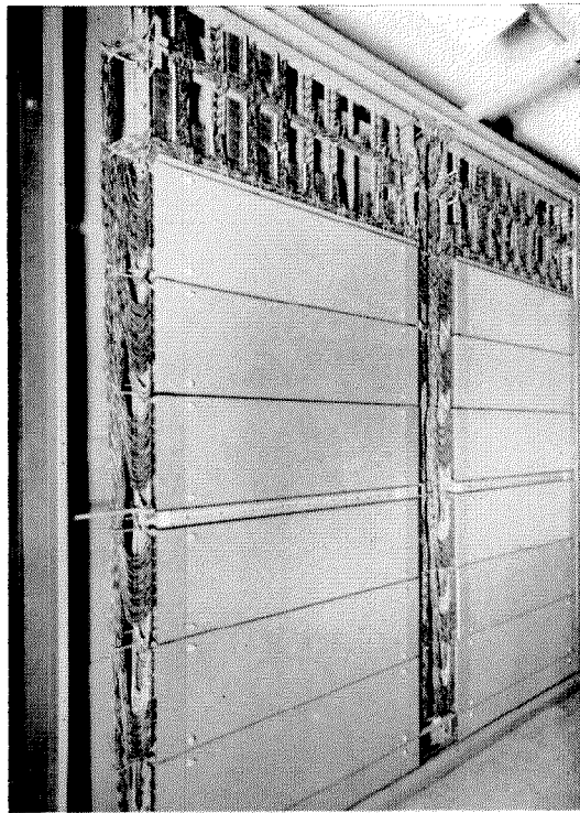
Figure 18—Bays of junctions and register finders.
