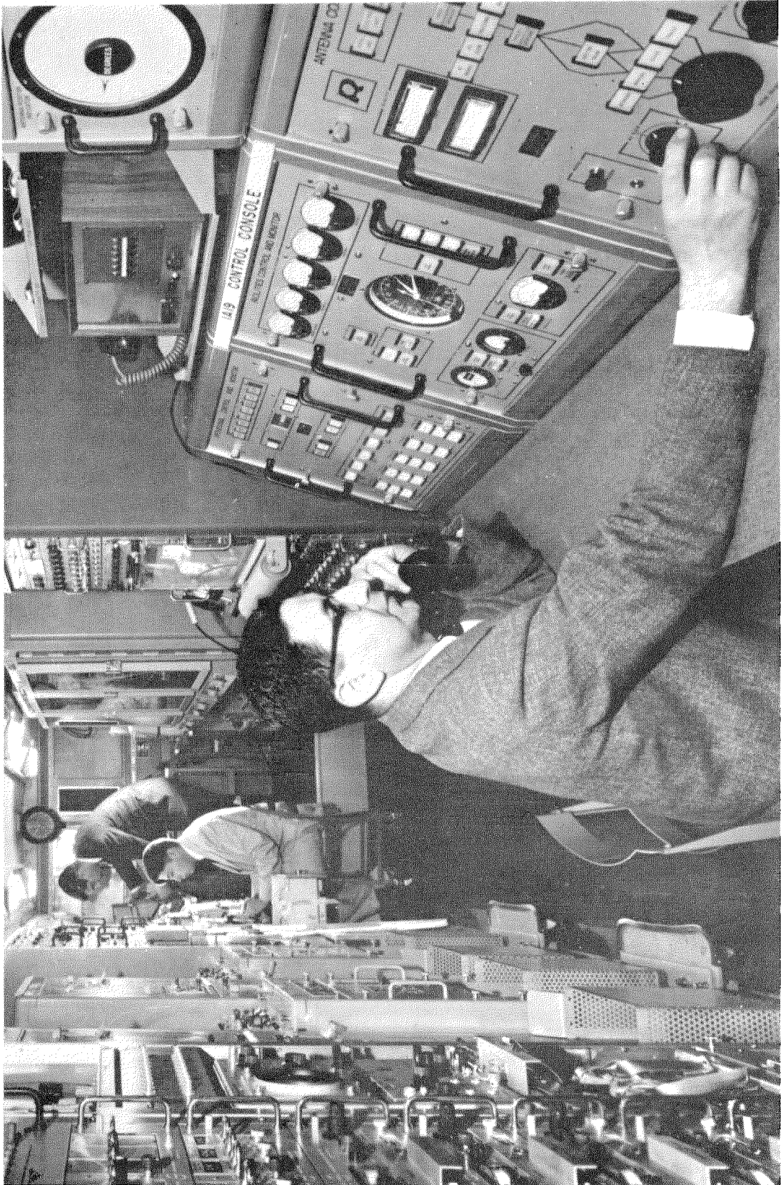
Figure 1—Courier satellite ground equipment for handling 340 000 words to and from the satellite during its 5-minute exposure to the ground station on each trip around the earth.
