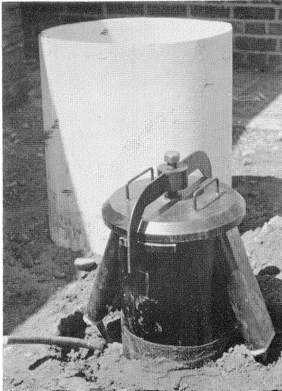
Figure 12—Repeater housing projecting from the ground.
