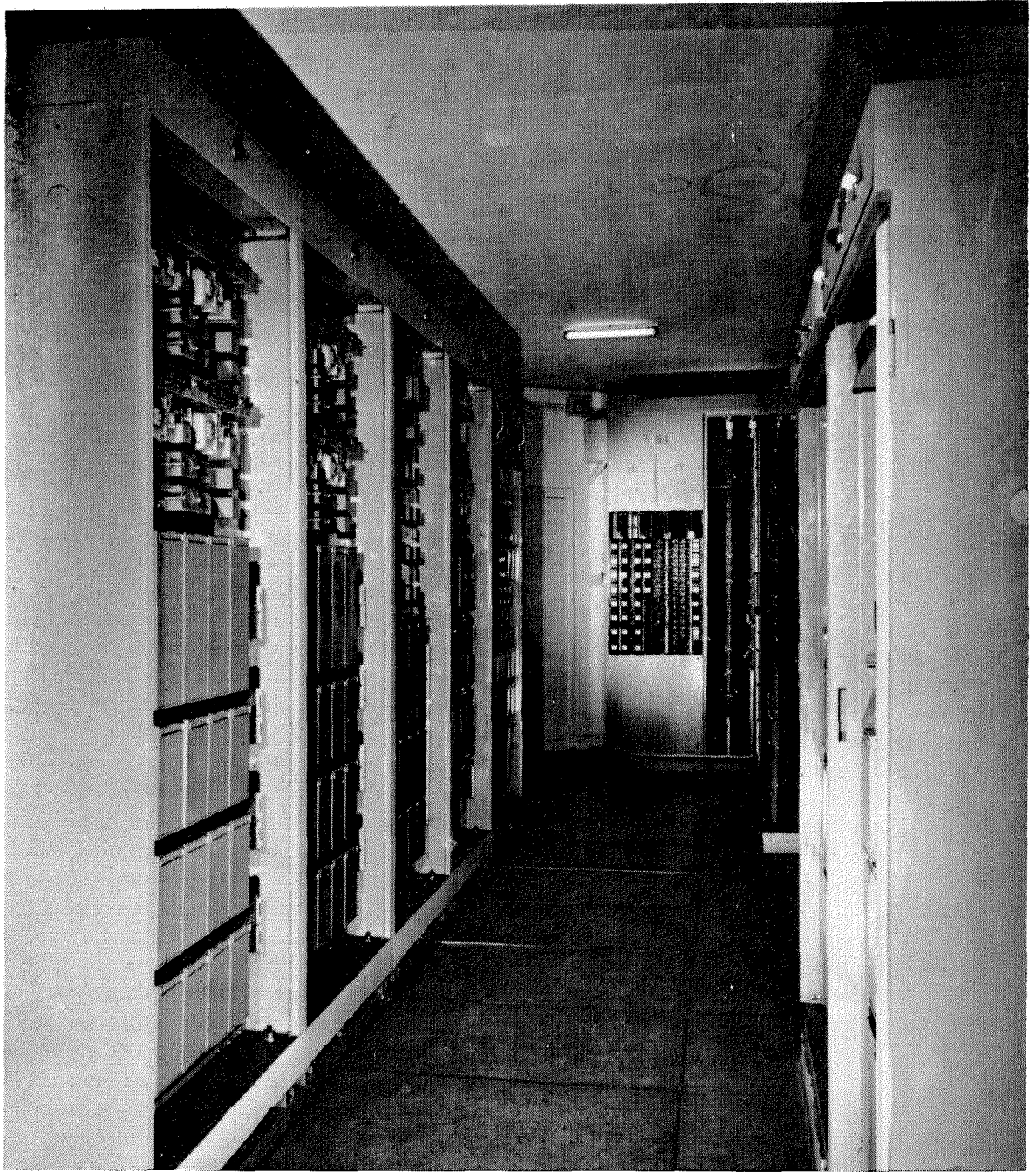
Figure 4—Racks of telecommunication switches at Algiers and terminations of cables to Arba.
