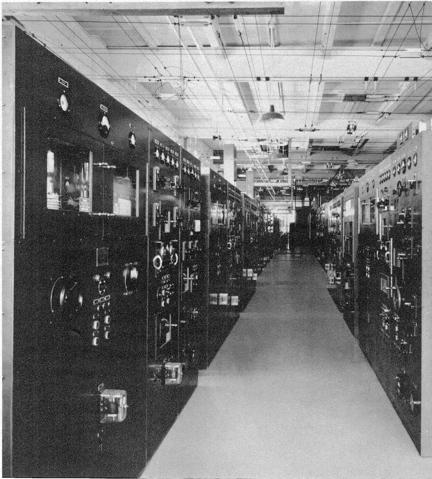
18. Two rows of high-power high-frequency transmitters at Brentwood. The grid of wires on the ceiling permits any of the 50 transmitters at the station to be connected to any of the outside transmission lines leading to the various antennas.
