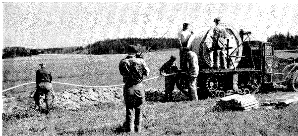
Figure 7—Rear view of vehicle showing mounting of cable reel and method of paying out cable into trench.
