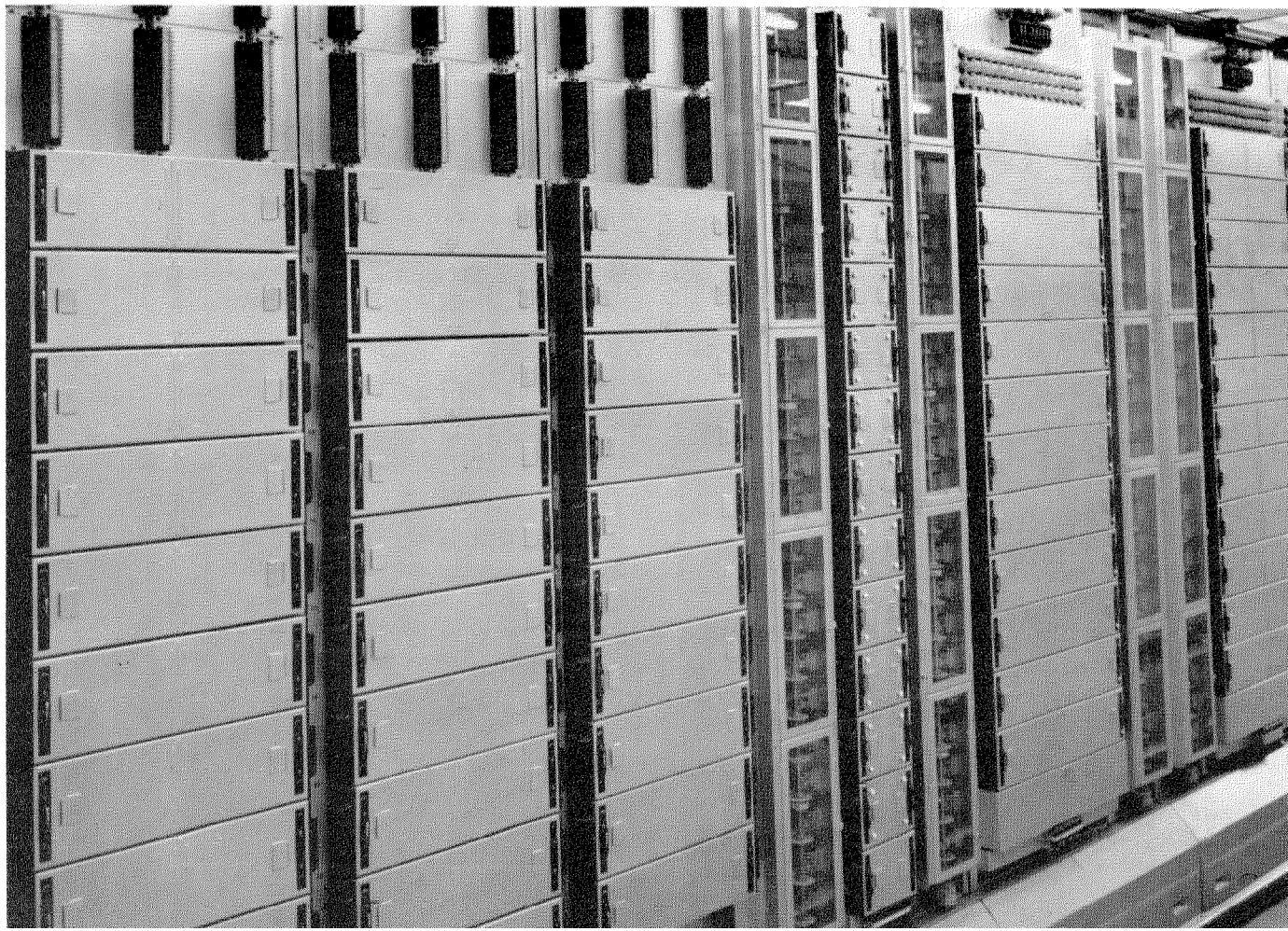
Figure 15—Part of switch rack mounting circuits for 200 subscribers' lines.
