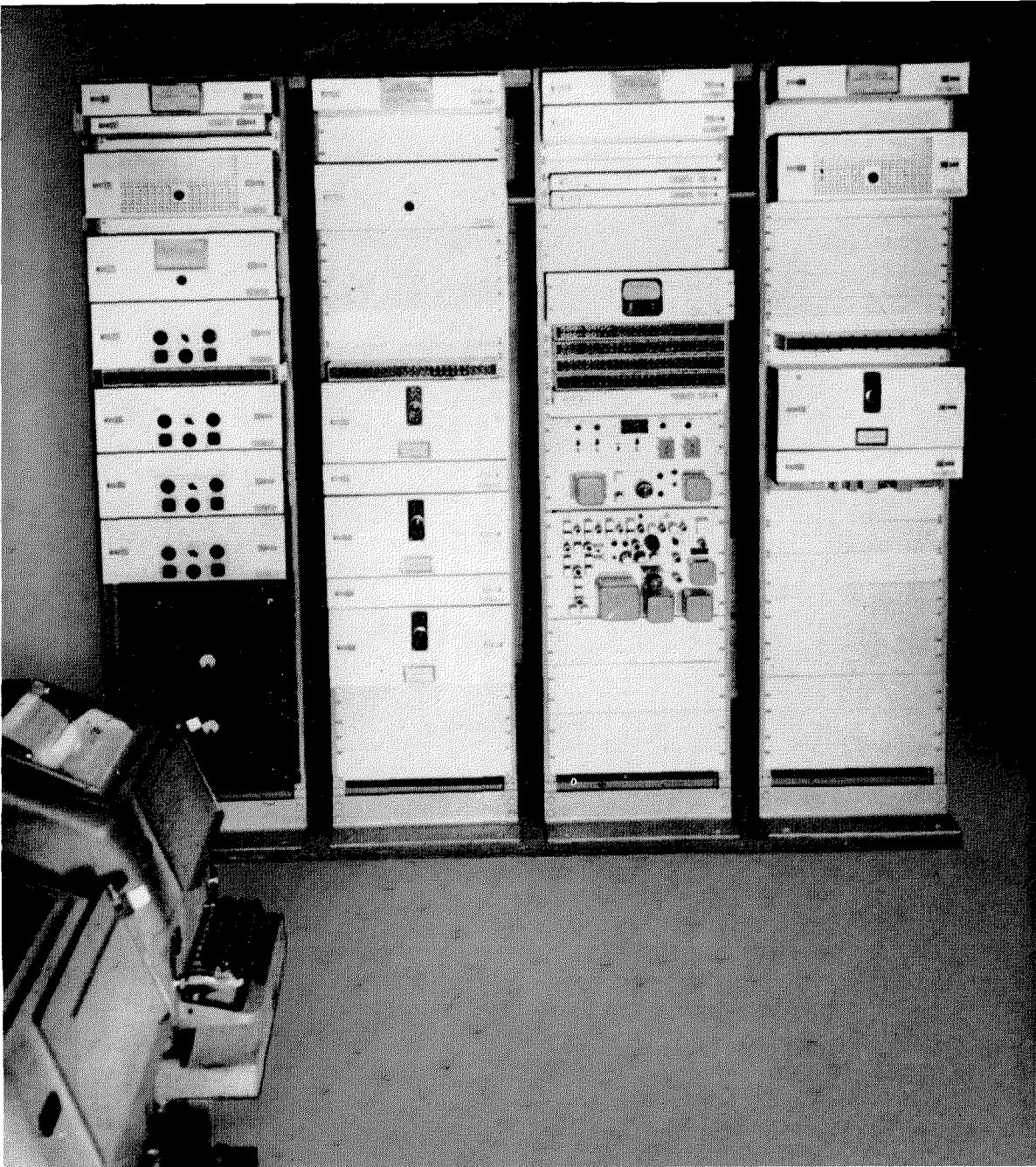
Figure 9—Telegraph carrier equipment at Charlotte Amalie.
