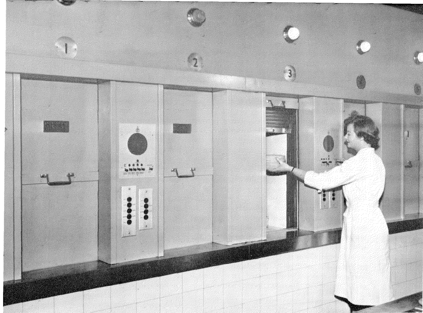
Completed installation showing lifts with intercommunication panels immediately above the lift-operation controls.
