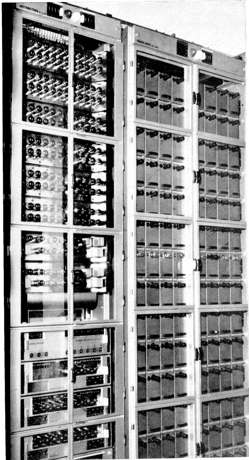
These two of the three bays house the pilots, distributors, amplifiers, and control circuits.
