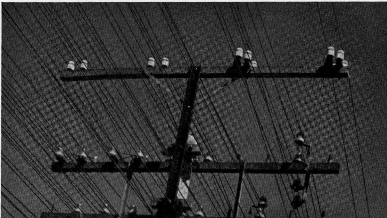
Figure 12—Typical crossarms, insulators, and transposition brackets. The zero crossarm carries 5.9-inch (15-centimeter) spaced wires on type-2 porcelain insulators mounted on H-15 -type transposition brackets. The first crossarm supports wires with 11.8-inch (30-centimeter) spacings; they are carried on double-petticoat alkaline-glass insulators mounted on both point- and drop-type transposition brackets.
