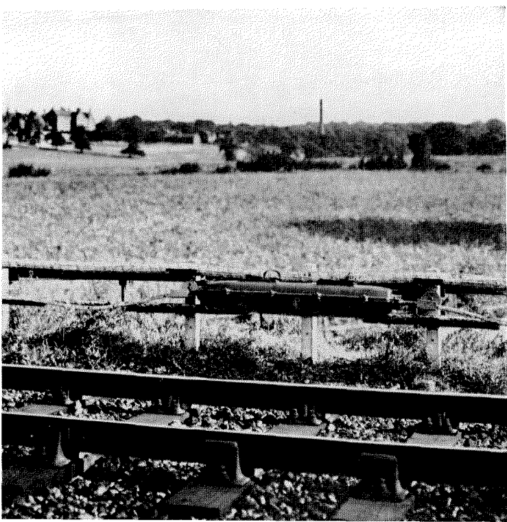
Figure 6—Pilot cables showing a loading-coil joint.
