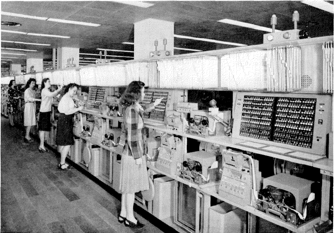
Push-button switching aisle in Philadelphia, Pennsylvania, office of Western Union Telegraph Company.
