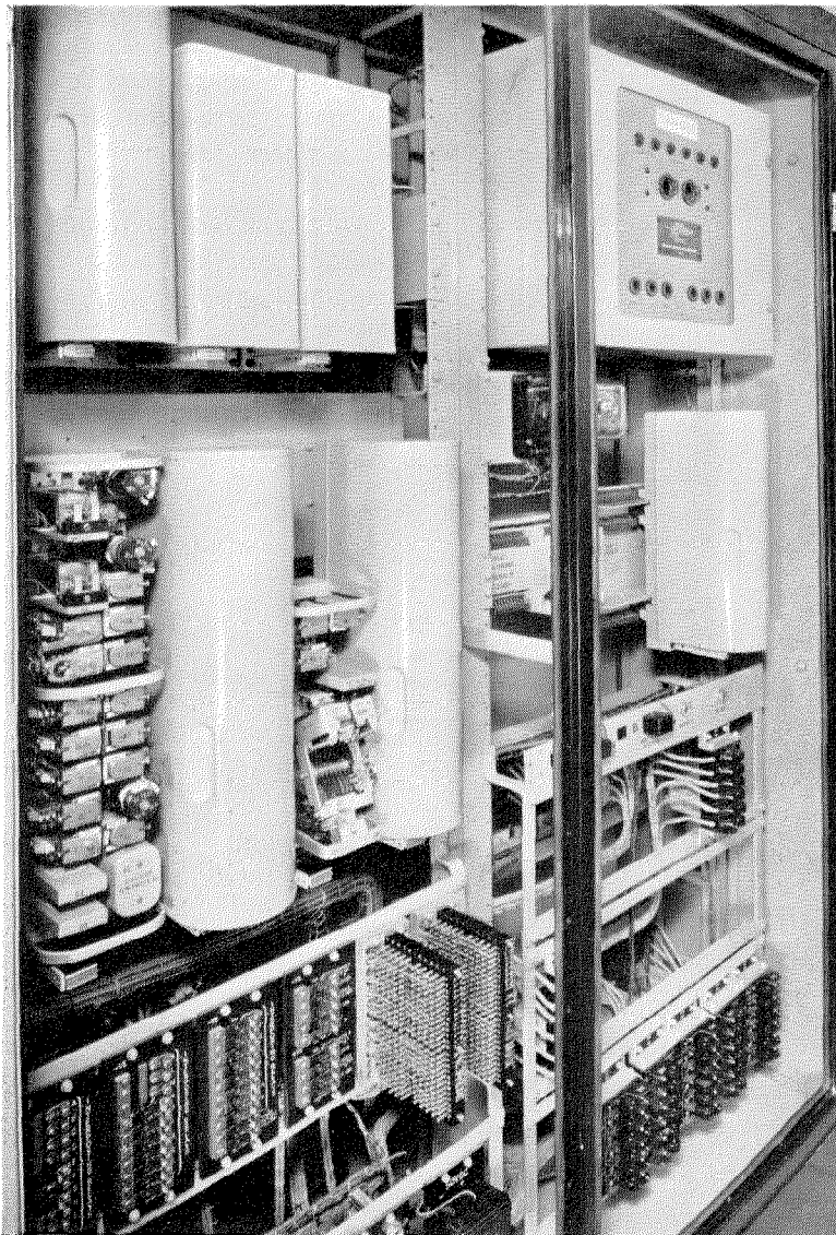
Figure 2—Supervisory apparatus of the type installed in substations. Jack-in panels permit rapid replacement of a faulty unit with a spare known to be in operating condition.
