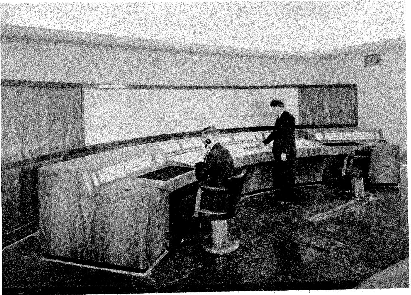
Figure 1—Control room at Chadwell Heath. The mimic diagram is just back of the curved control desk.
