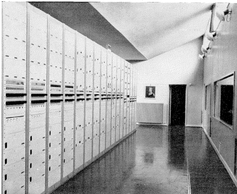
Fig. 2—Part of the amplifier room.
