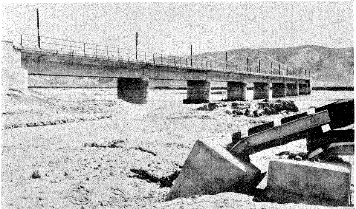
View of the bridge after the flood. Remains of one of the H structures are in the right foreground. All land between the end of the bridge and the distant right was washed out. The poles lashed to the bridge railing support the emergency lines.
