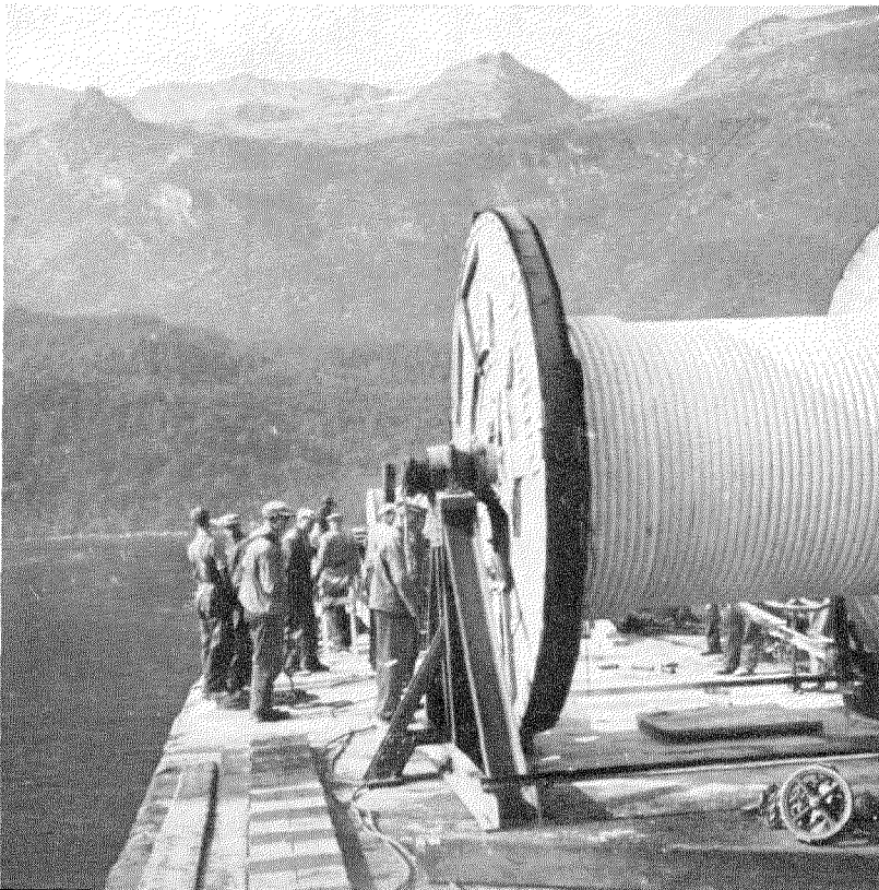
Reel of cable on a cable-laying lighter. The terrain at a typical deep fiord is shown here.
