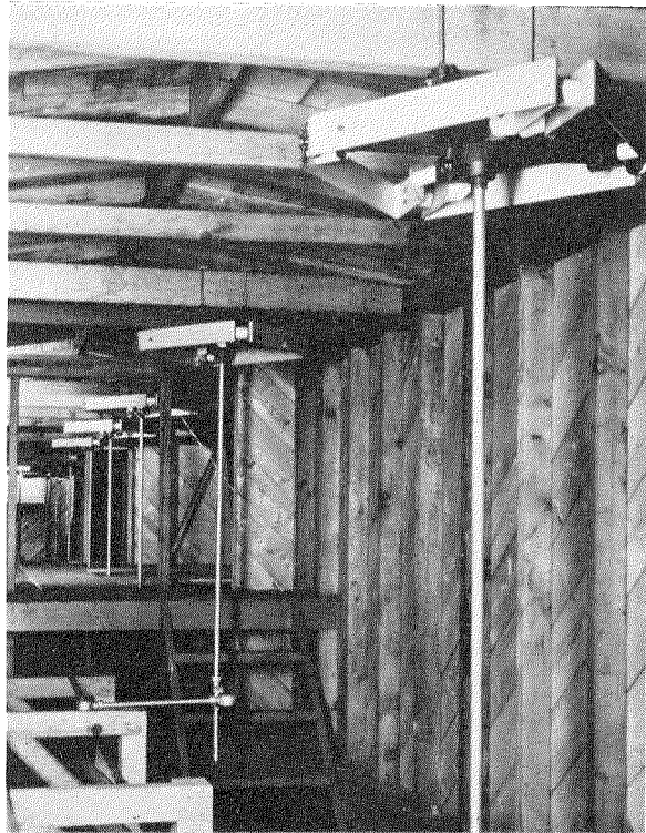
Interior view of the localizer house for a Civil Aeronautics Authority installation.
