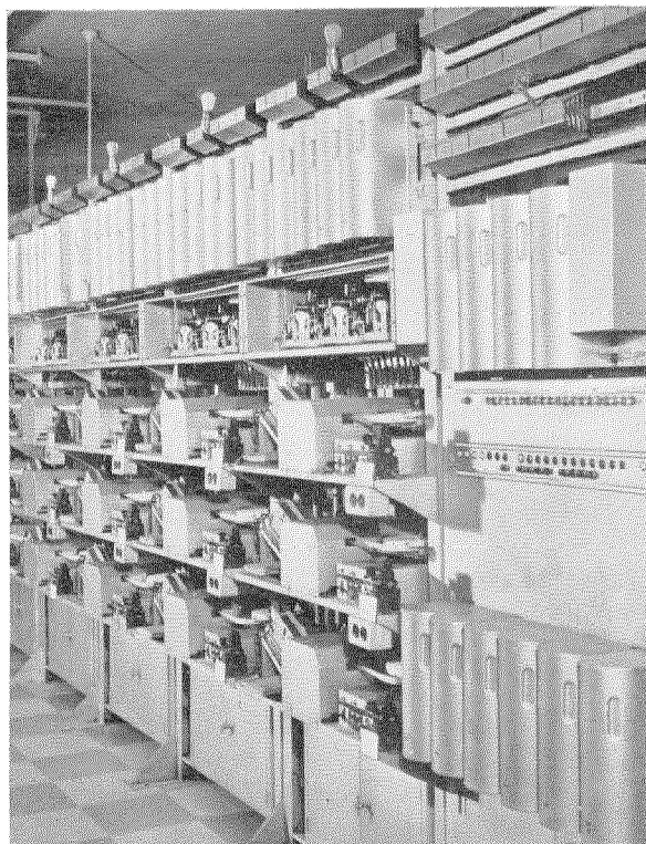
Fig. 4—Varioplex Central Office equipment common to all connections.
