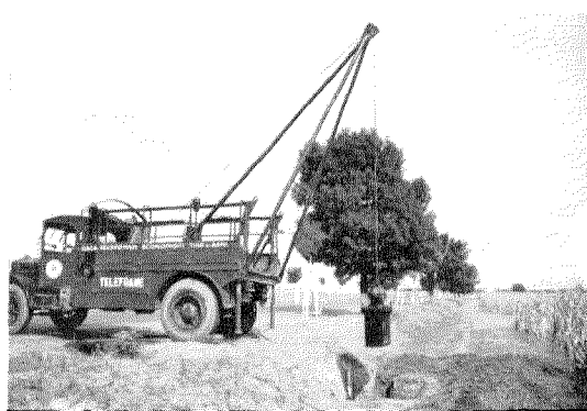
Placing Loading Coil Case in Position. The loading coil case contains 60 units (i.e., 120 side circuit and 60 phantom coils) for loading the 60 voice frequency multiple twin quads. It weighs approximately 700 kg (14 cwt.).
