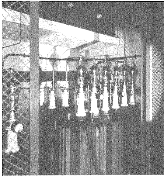
Fig. 17—One of the Hot Cathode Mercury Vapour Rectifier Units supplying the High Tension to the Power Stages of the Transmitter.
