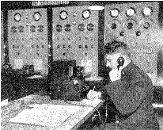
Fig. 4—Radio Telephone Switchboard Room at Headquarters.
