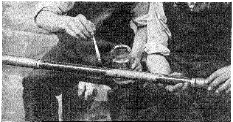
Figs. 2 and 3—Two stages in the fabrication of a styrene joint by the "cold process" using pre-polymerised styrenated paper.
