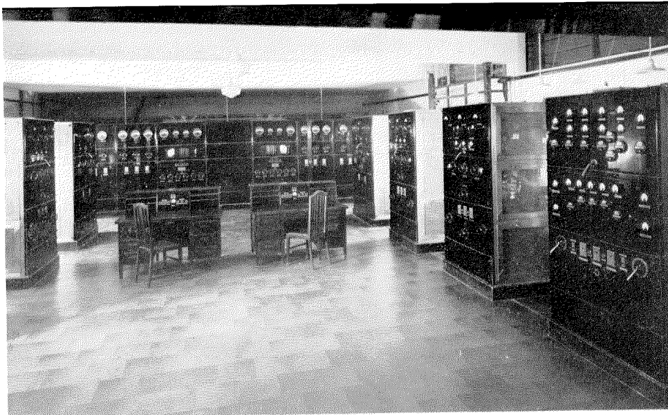
Figure 5—Transmitter Hall Showing Twin Transmitters on Either Side and Power Control Board at End.
