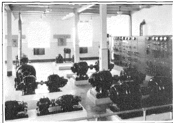
Power Room, Principal Central Office.
