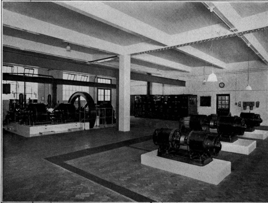
General View. Power Room, Derby
