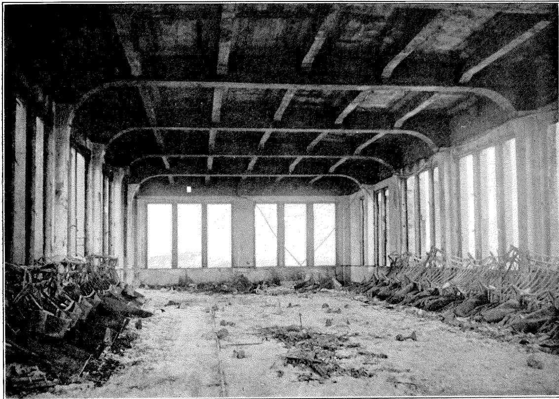
Figure 11—Ruins of Switching Room After Fire in Telephone Central Hamacho, Tokio
