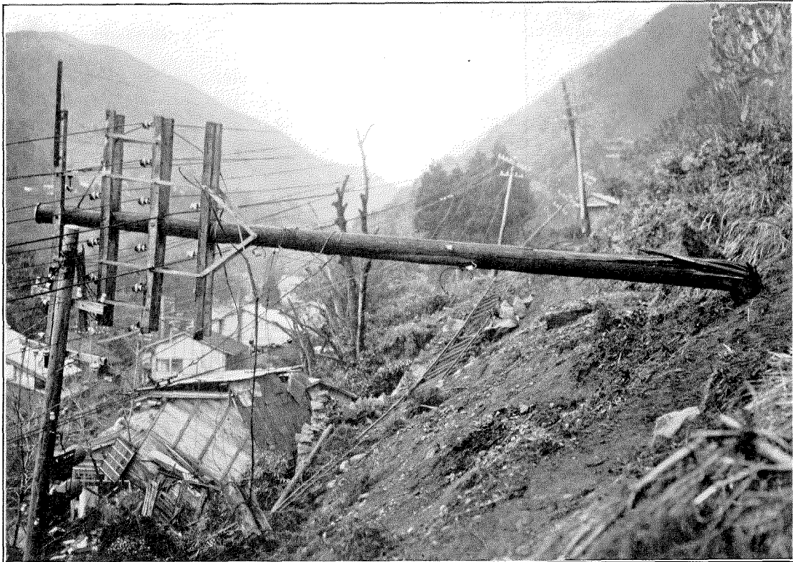
Figure 18—Disaster of Pole Line Near Hakone. Longer Poles are for Power and Lighting. Smaller Ones for Telephone
