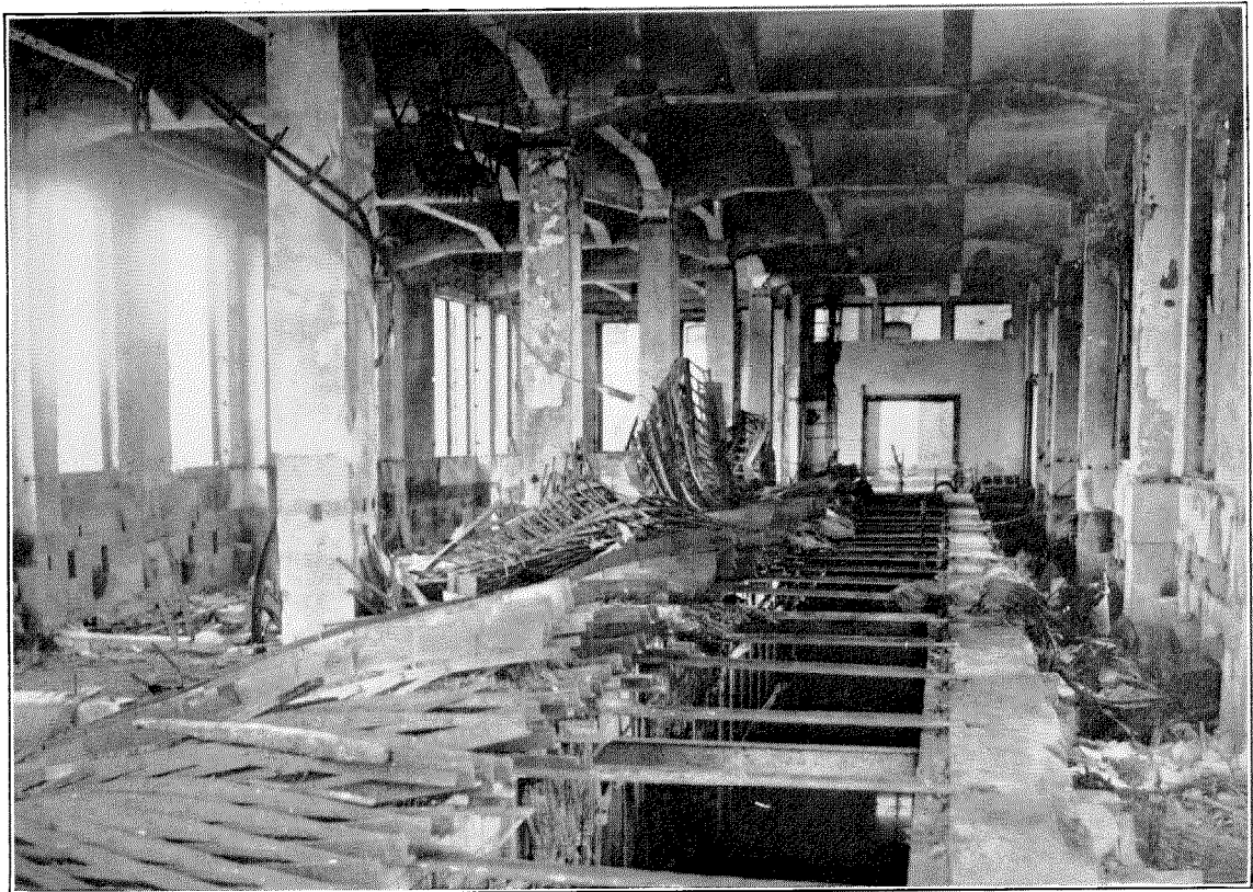
Figure 12—Ruins of M. D. F. and Office Manhole After Fire in Telephone Centrals Hamacho and Horidome, Tokio
