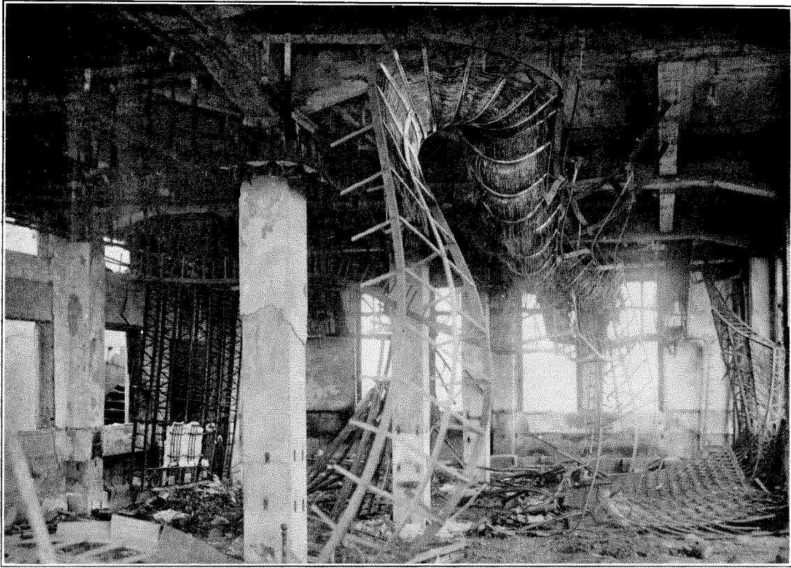
Figure 10—Ruins of Cable Room After Fire in Telephone Central Horidome, Tokio
