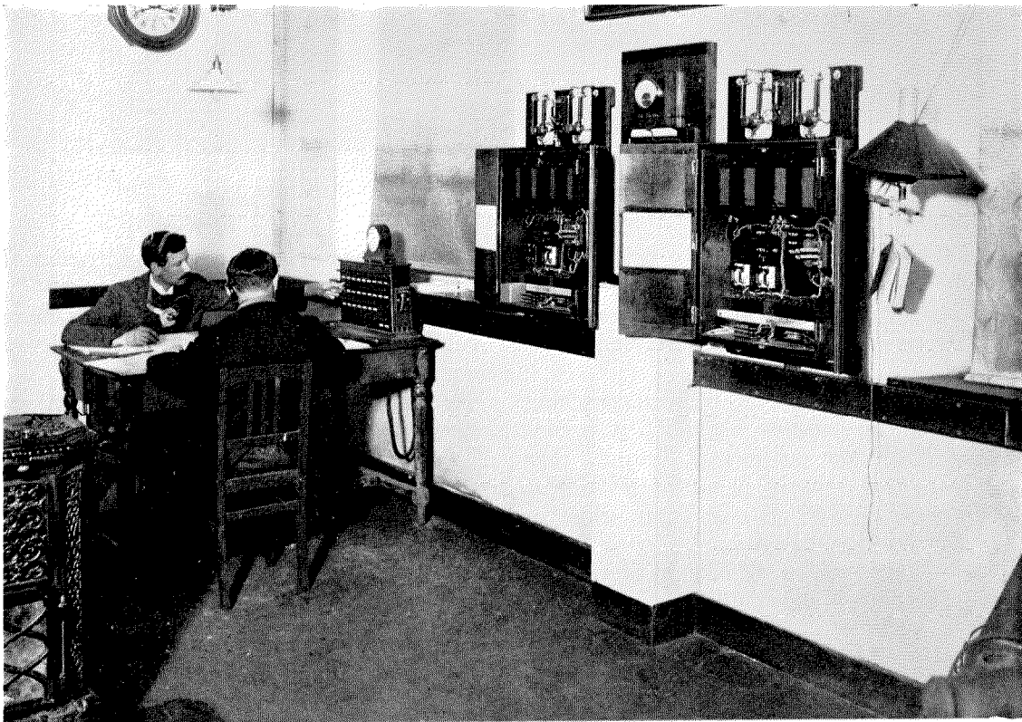
Figure 11—Dispatcher's Office—Bruxelles Nord, Belgium
